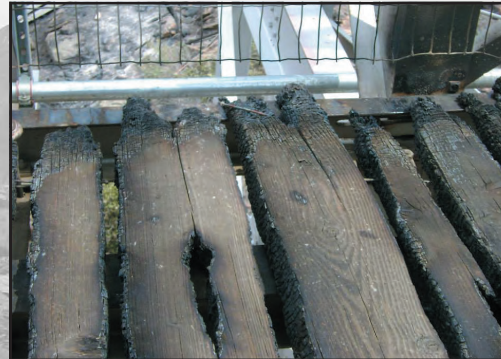
Some of the bridge planks that were scorched during the fire. Courtesy Photo
