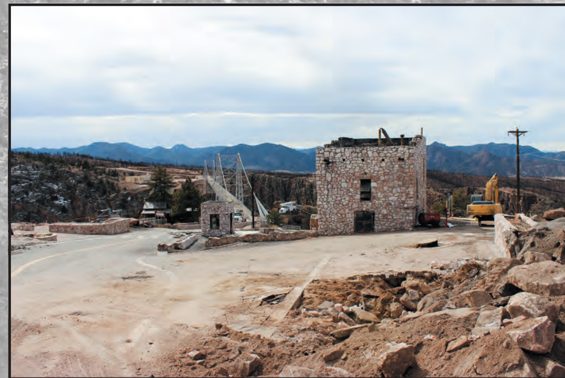
The incline railway cable house after the fire.
